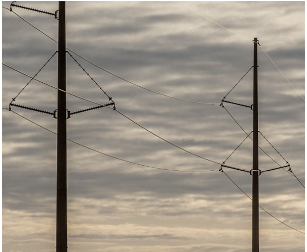
Montana-Alberta Tie-Line | Enbridge
